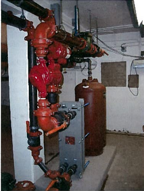
Figure 2. Snow melt heat exchanger in the city's Heat Exchanger building.
